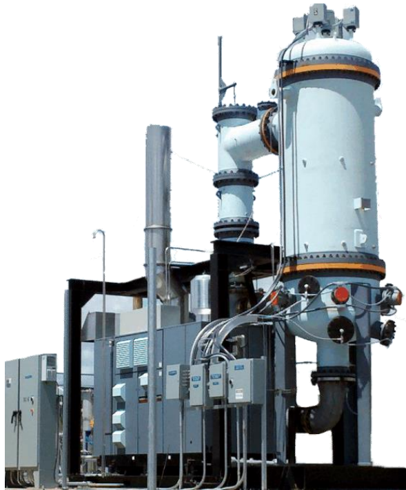
Image 1 shows an Ener-Core Power Oxidizer assembly. The white vessel provides extended residence time over standard gas turbines.
